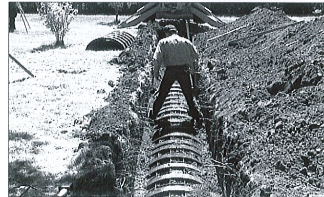
Pack down the fill by walking along the edges of the trench.
